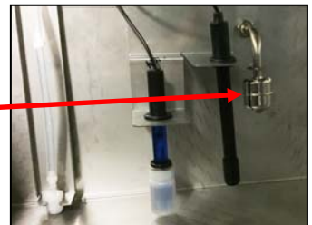
Fig. 2 Float switch/sensor; left side of reservoir; shuts off water once filled to proper level
